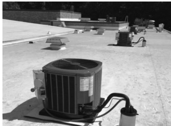
Rooftop Condensing Unit for Air Conditioning at Cornell
