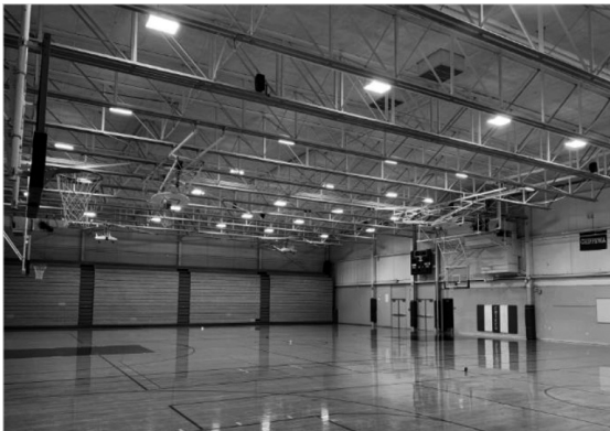
Chippewa Gymnasium LED Lighting
